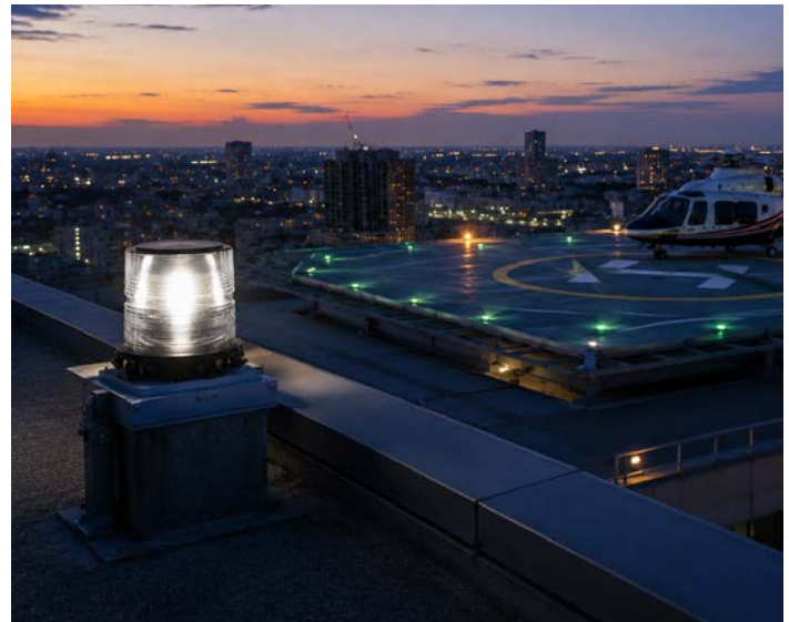
Flight Light recommends that heliport beacon placement be evaluated for site-specific requirements in consultation with a local FAA representative.
