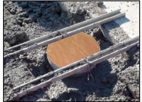
Installed Base Can
